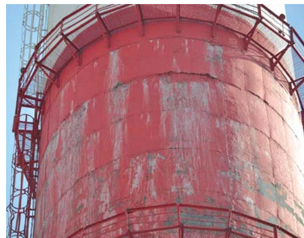
Fig. 4. Leaching process of free lime through weakened concrete sections
